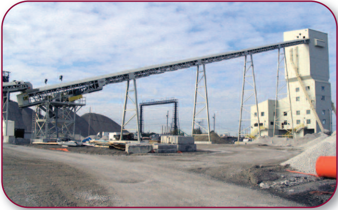
42" x 326' Stationary Feed Conveyor
