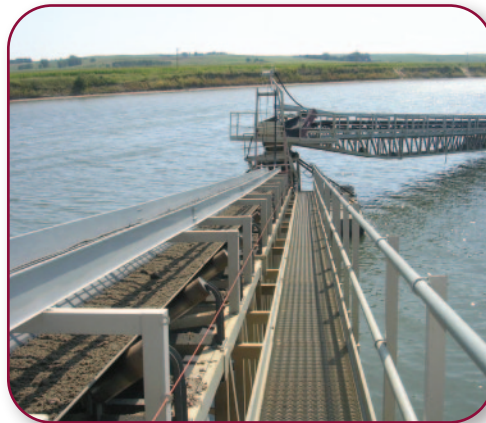
Multiple 36" x 100' Floating Pontoon Conveyors
