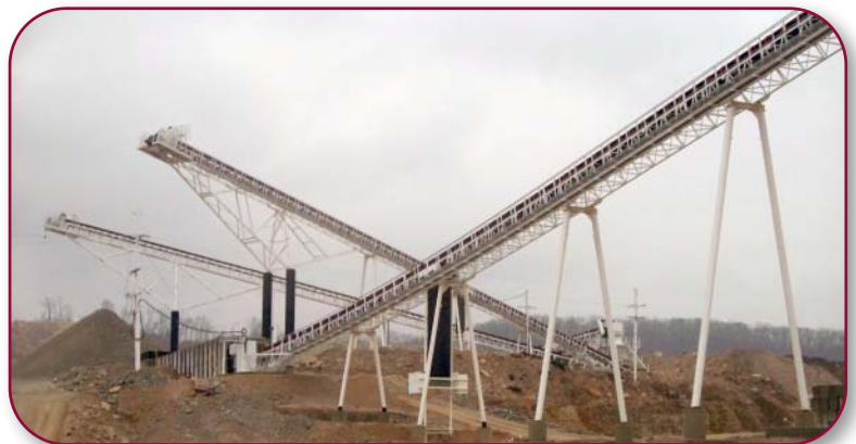
42" x 274' (2) Stationary Surge Pile Conveyors 42" x 704' Tunnel Feed Conveyor (Front)
