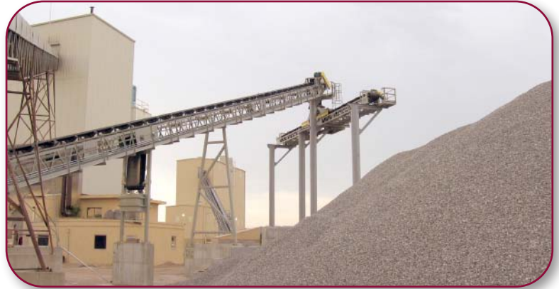
30" x 200' Stationary Truck Unloading Conveyor feeding two 30" x 31' Stationary Conveyors
