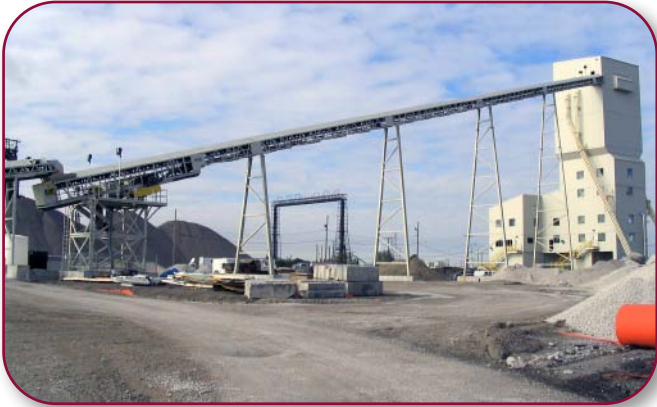
42" x 326' Stationary Plant Feed Conveyor
